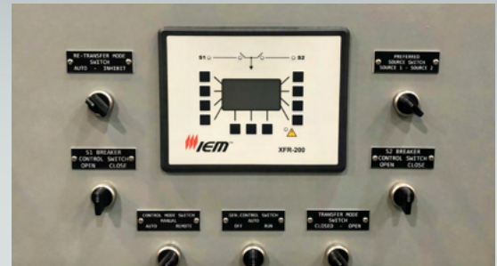
Transfer Switch XFER-200 controller and LCD display
